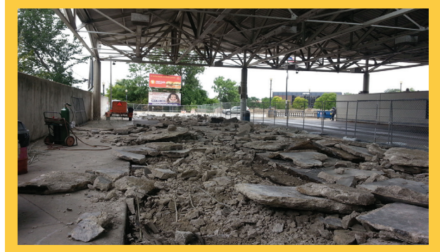
In 2015, Pace began a major mid-life renovation to the Pace Transportation Center in Elgin.
