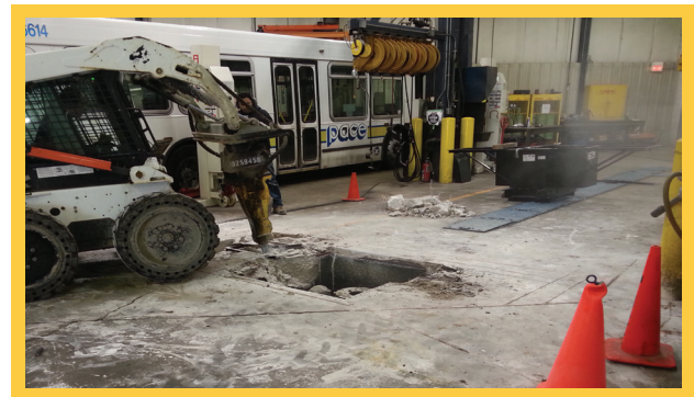
Pace replaced the in-ground lifts at Northwest and North Shore Divisions.
