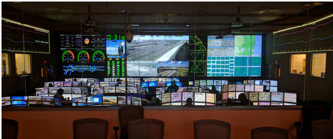
One of Florida Department of Transportation's Regional Transportation Management Centers ( www.fdot.gov ).
