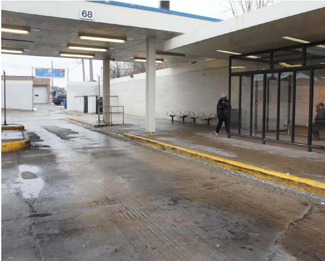
Photo 2: Some staining (a de minimis condition) is visible on the pavement in this view of Berth 68, looking north.
