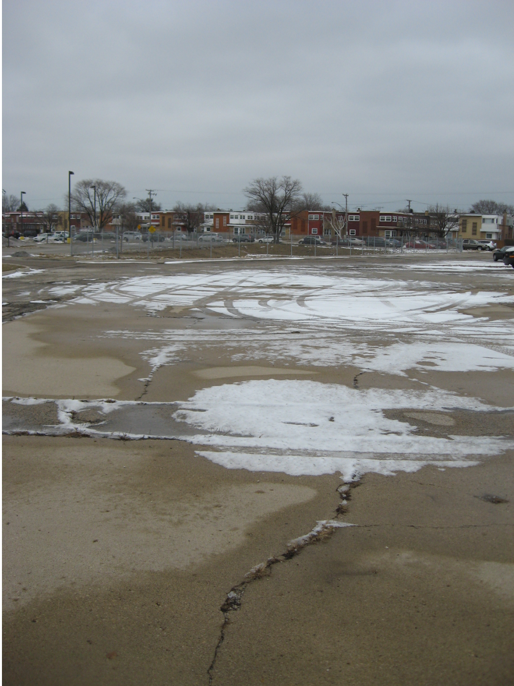
Photo 3: The former pump islands are visible in the pavement of the Niles Truck Rental parking lot, located immediately east of the proposed northbound Dempster Street Station location, looking east.
