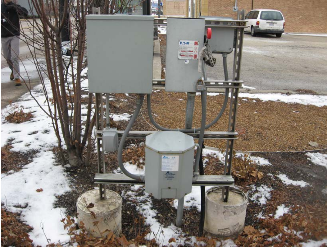
Photo 5: Closer view of the electrical panels located near the existing southbound station, looking south. The building visible in the background is occupied by United Transmissions, which was listed on the UST and RCRA NON GEN databases.
