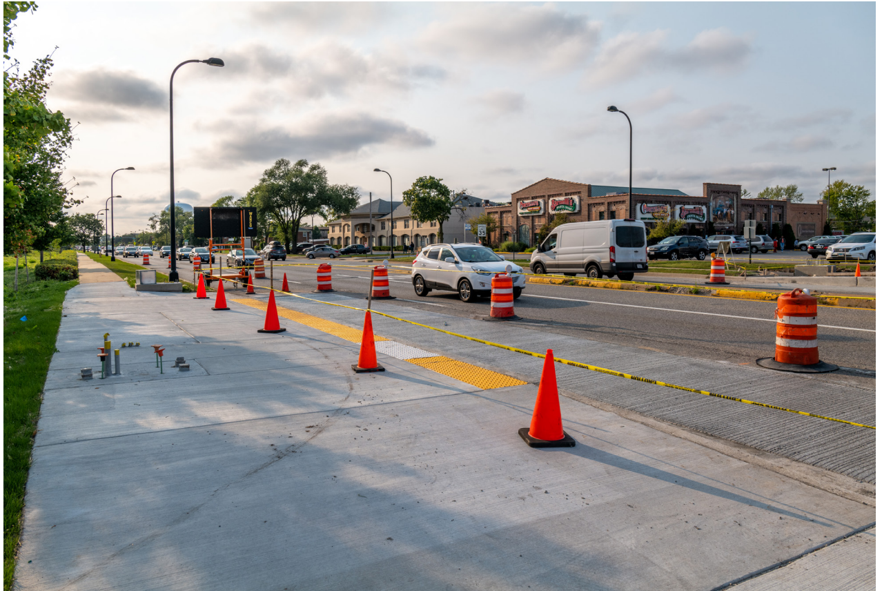
Station under construction on the Pulse Dempster Line | Photo by Andy Ryan
