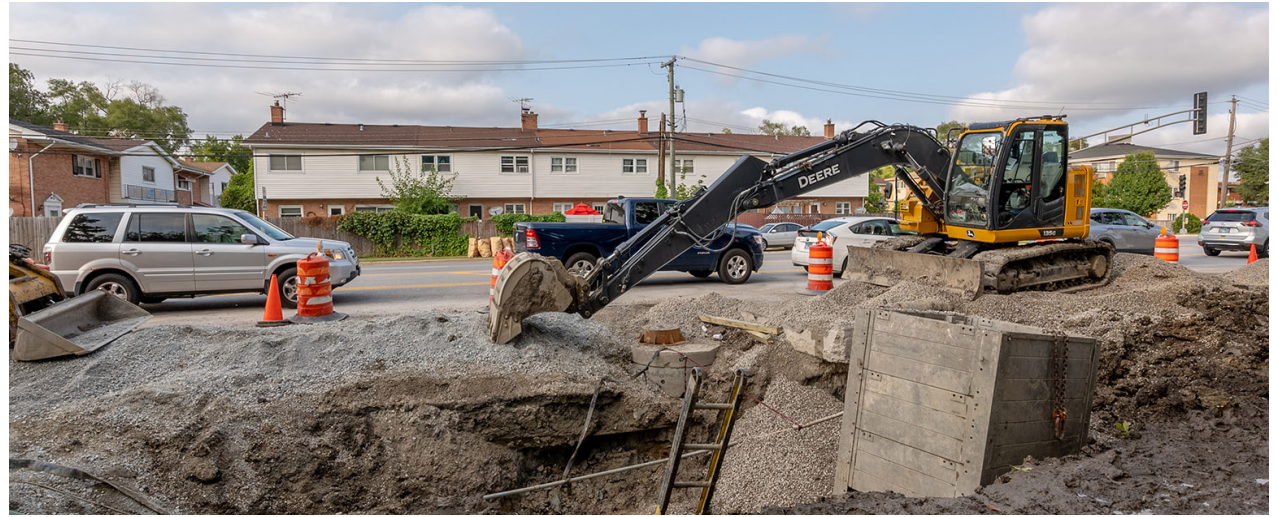
Station under construction on the Pulse Dempster Line | Photo by Andy Ryan
