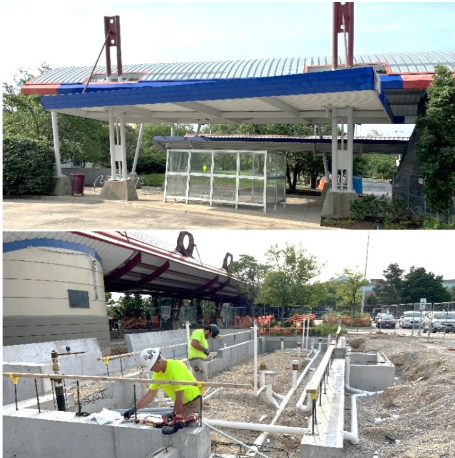
Photo: Top to Bottom, In progress Northwest Transportation Center and new ADA Transfer Facility
